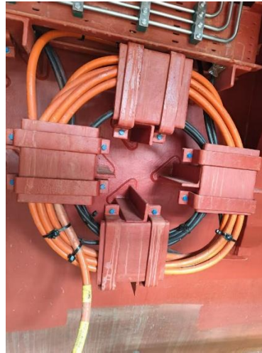
Figure 26: Cable overlength solution example at lower riser balcony
