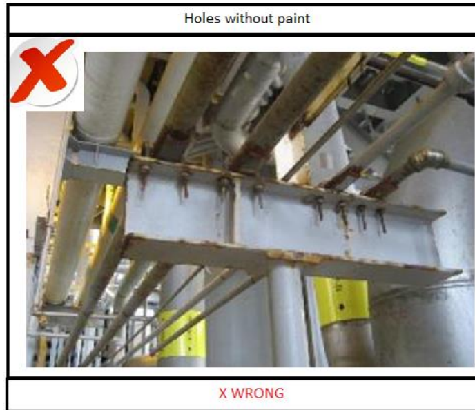
Figure 8 – Hole for bolts drilled with no precaution for not damaging the paint and with no preservation during assemble
