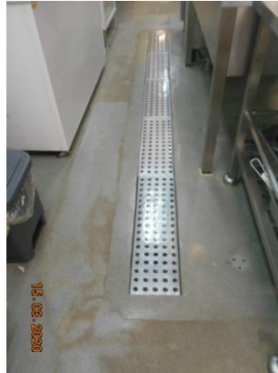
Figure 4. Grilles used for draining water from kitchen floor.
