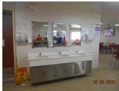
Figure 13. Sinks for hand hygiene in the messroom.
