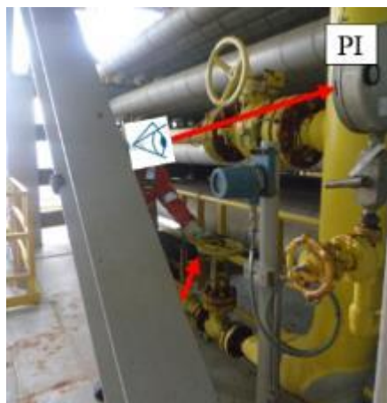
Figure 7. Module support beams restrict access to valves and location of the IP indicator concerning the valve.
