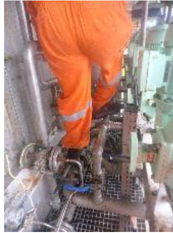
Figure 4. Valves installed in a place where access requires permanence on pipes and equipment.
