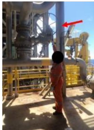
Figure 15. Valve installed above the operator's range.
