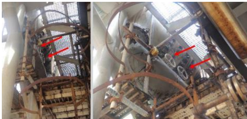
Figure 25. Improper position of category 1 valves.
