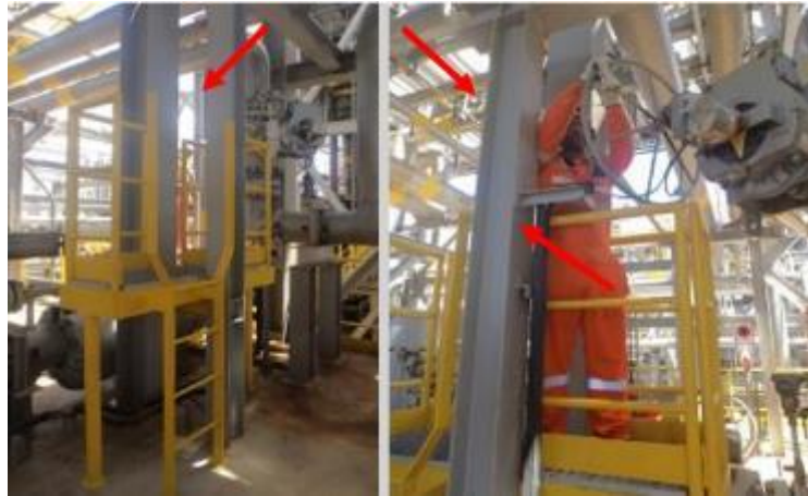
Figure 24. Valve with access by fixed platform, but with restricted access
