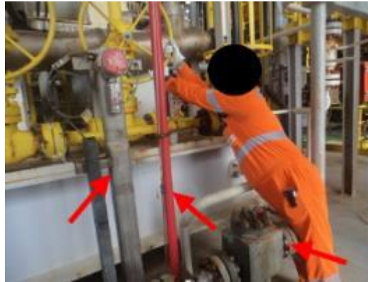
Figure 14. Difficulty in accessing the valve due to obstacles in its surroundings.
