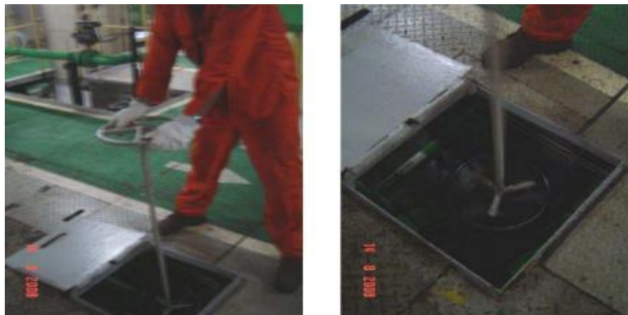
Figure 8. Mobile device to operate valves positioned below the floor.
