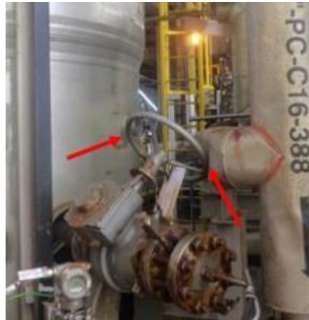
Figure 6. Lack of space around handwheel and inadequate valve position does not allow operator access.
